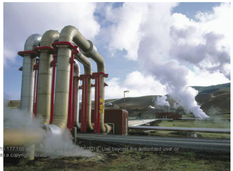
▼ FIGURE 9-47 GEOTHERMAL Geothermal plant near Krafla, Iceland.
