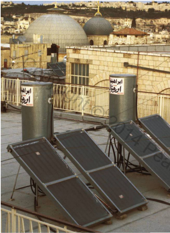
▲ FIGURE 9-48 SOLAR PANELS Solar panels installed on apartment rooftops in the Old City of Jerusalem are used to heat water, which is stored in the adjacent tanks. The domes are the Church of the Holy Sepulchre, built at the site where Jesus is thought to have been crucified, buried, and resurrected (see Chapter 6).
